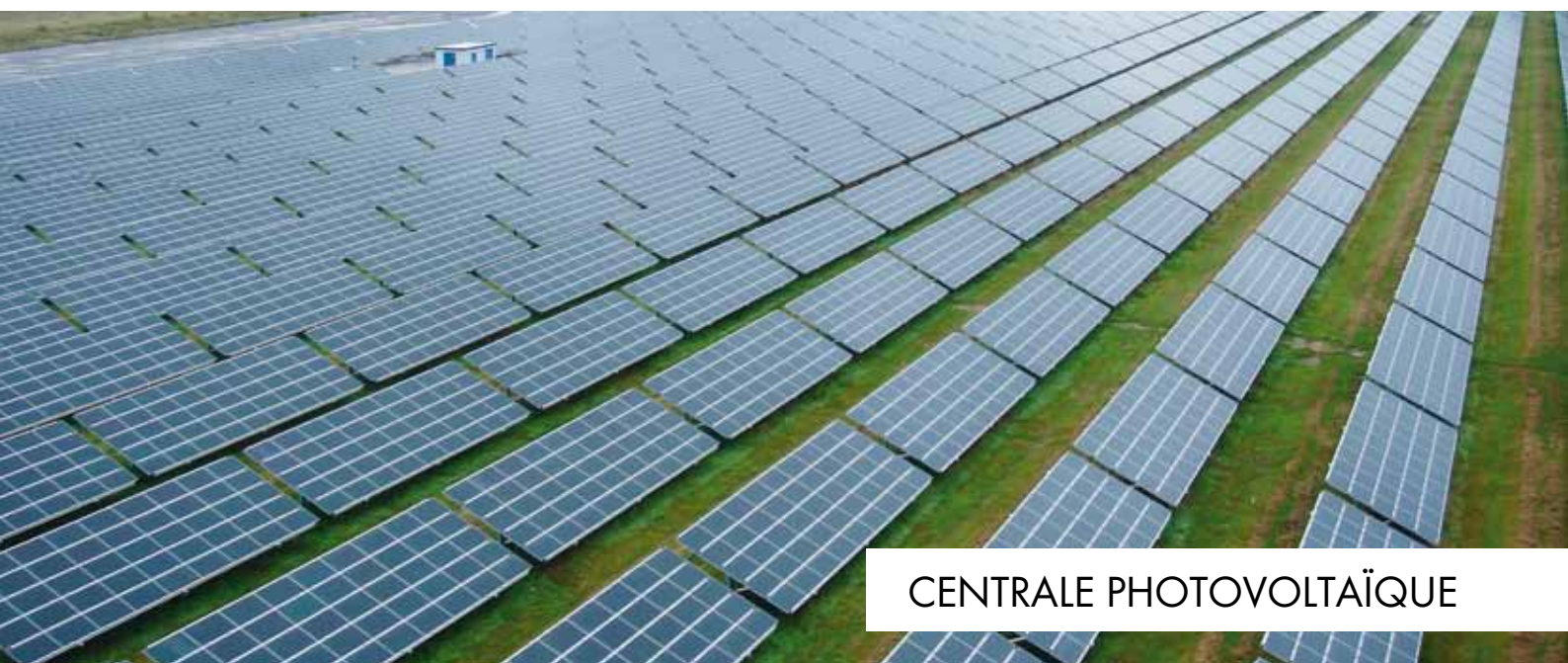
INSTALLATION PHOTOVOLTAÏQUE INDUSTRIELLE
